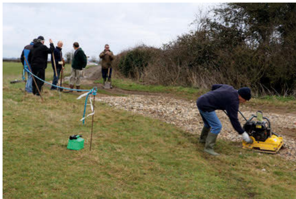
Volunteers repair the access road at Vale of White Horse Gliding Club (Kevin Hale)
